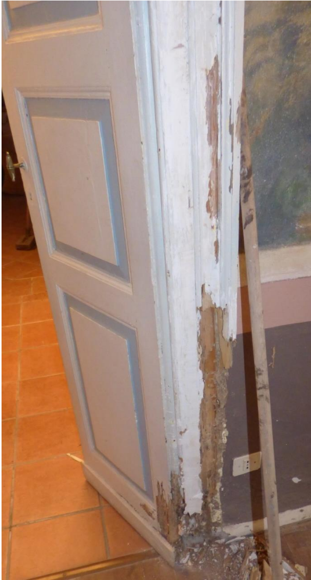
Figure 2. Termite damage in wooden door framing in Spinetta Marengo.
